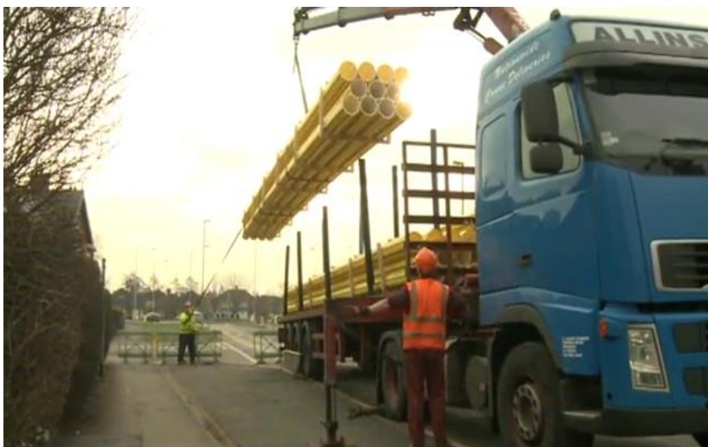
Figure 18 – Unloading smooth tubes into bars, with a munck truck and a guide man
